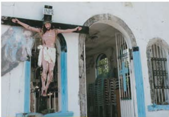
A chapel in need of repair
